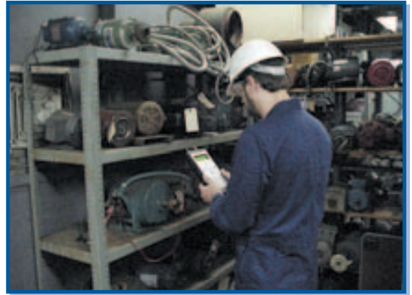
Testing spare motors to confirm their status insures against installing a faulty motor.
