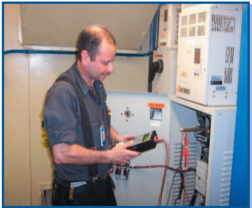
A 2-minute test from the MCC evaluates the windings, cabling, and connections through even hundreds of feet of cable.
